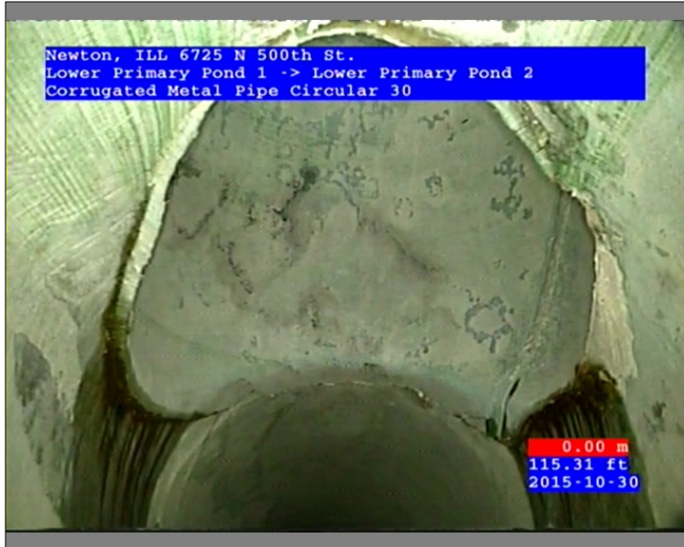
Photo: 45602-103015-01-AECOM Denver-3-30102015145614_B.JPG 115.32FT, Tap Factory Made, at 12 o'clock, -, within 8 inches of joint: YES, 30" / Upper Primary
