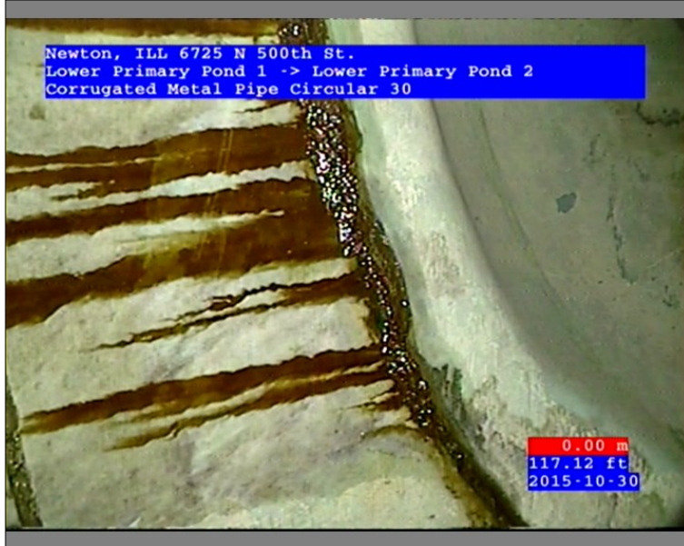
Photo: 45602-103015-01-AECOM Denver-3-30102015145940_A.JPG 117.12FT, Infiltration Weeper, from 08 to 11 o'clock, within 8 inches of joint: YES
