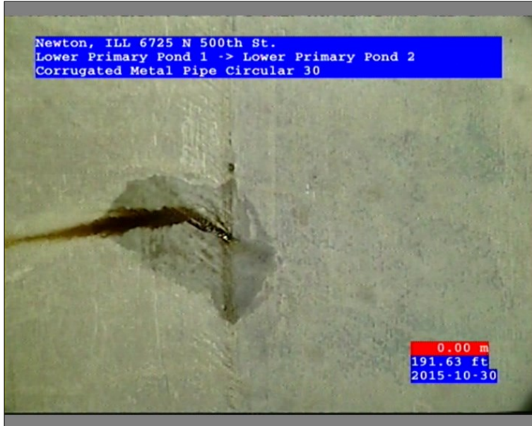
Photo: 45602-103015-01-AECOM Denver-3-30102015150655_A.JPG 191.63FT, Infiltration Weeper, at 09 o'clock, within 8 inches of joint: YES
