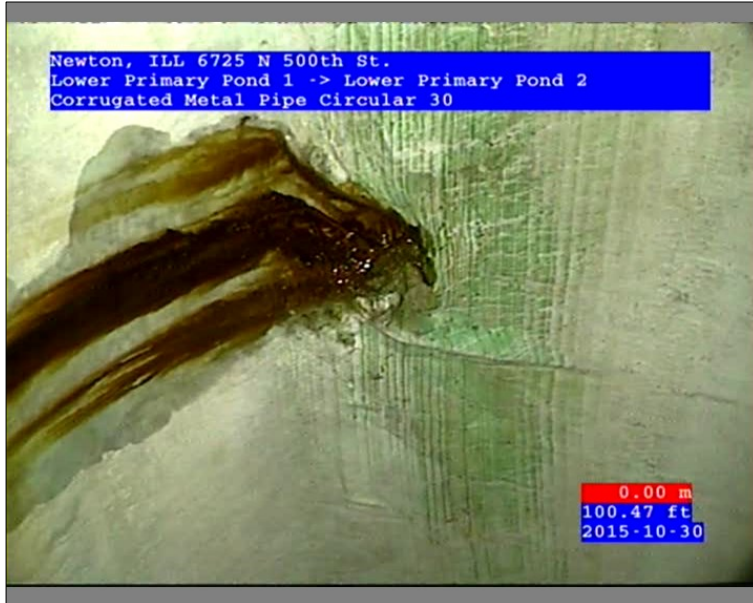
Photo: 45602-103015-01-AECOM Denver-3-30102015145428_A.JPG 100.47FT, Lining Failure Other, at 10 o'clock, within 8 inches of joint: YES / Leak
