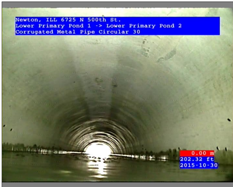
Photo: 45602-103015-01-AECOM Denver-3-30102015150946_A.JPG 202.32FT, General Observation / Reached Clients Needed Footage, Sediment Was Getting Thick
