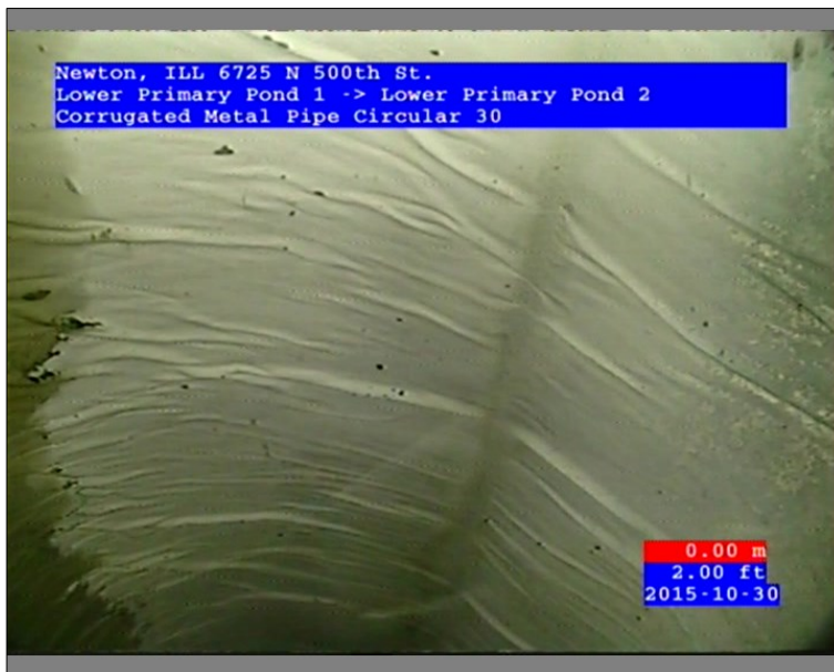
Photo: 45602-103015-01-AECOM Denver-3-30102015152117_A.JPG 2FT, General Observation / Crease
