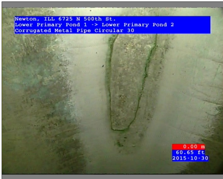
Photo: 45602-103015-01-AECOM Denver-3-30102015144916_A.JPG 60.65FT, General Observation / Air Pocket
