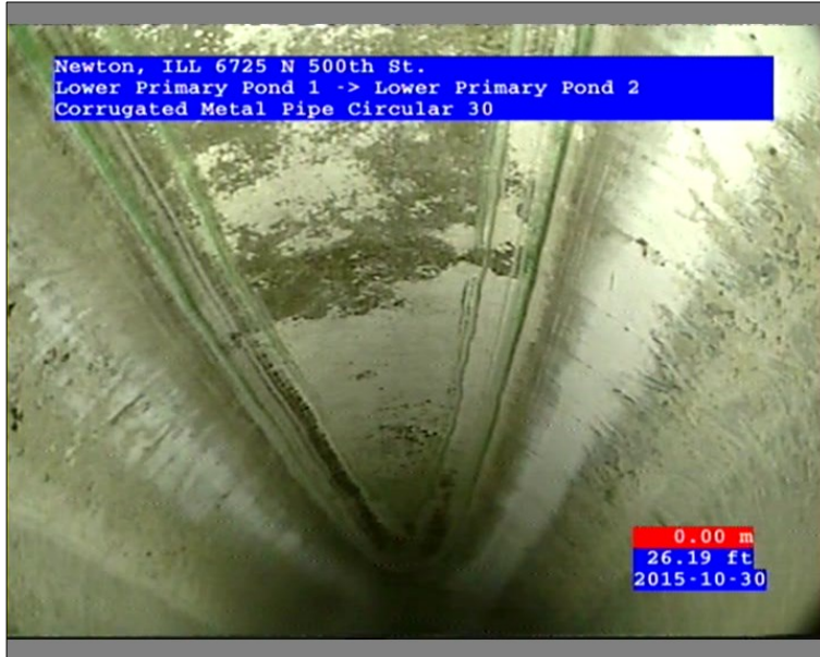
Photo: 45602-103015-01-AECOM Denver-3-30102015151901_A.JPG 26.19FT, General Observation / Air Pocket
