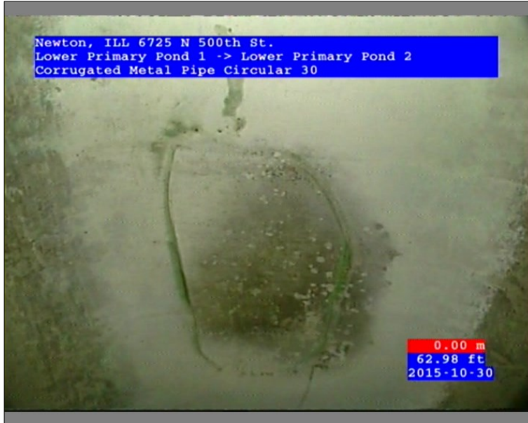
Photo: 45602-103015-01-AECOM Denver-3-30102015144950_A.JPG 62.98FT, General Observation / Air Pocket
