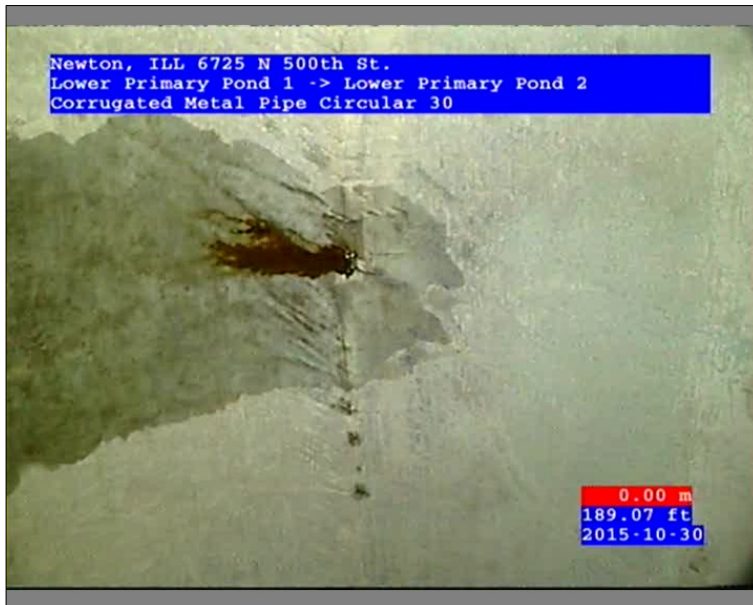
Photo: 45602-103015-01-AECOM Denver-3-30102015150617_A.JPG 189.07FT, Infiltration Weeper, at 09 o'clock, within 8 inches of joint: YES
