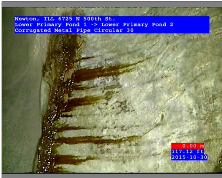
Photo: 45602-103015-01-AECOM Denver-3-30102015145847_A.JPG 117.12FT, Infiltration Weeper, from 12 to 03 o'clock, within 8 inches of joint: YES
